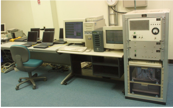
Figure 3: Experimental GBAS ground station main site From right: VDB transmitter, WS and PCs
